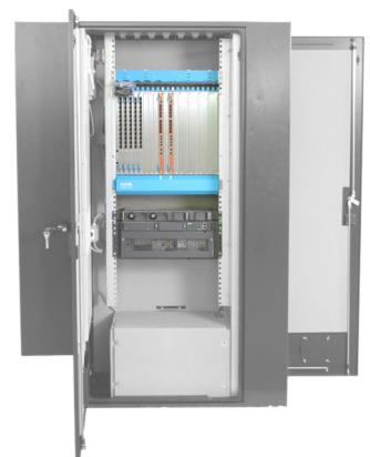
Deployment in street cabinets
